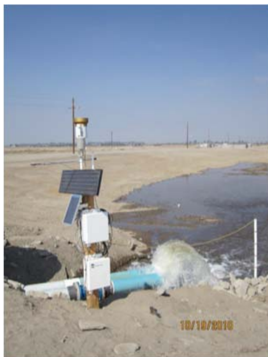
Figure 3. The new CENS-CITRIS managed aquifer recharge network (MARnet) prototype presently installed at the Fresno city wastewater treatment facilities.
