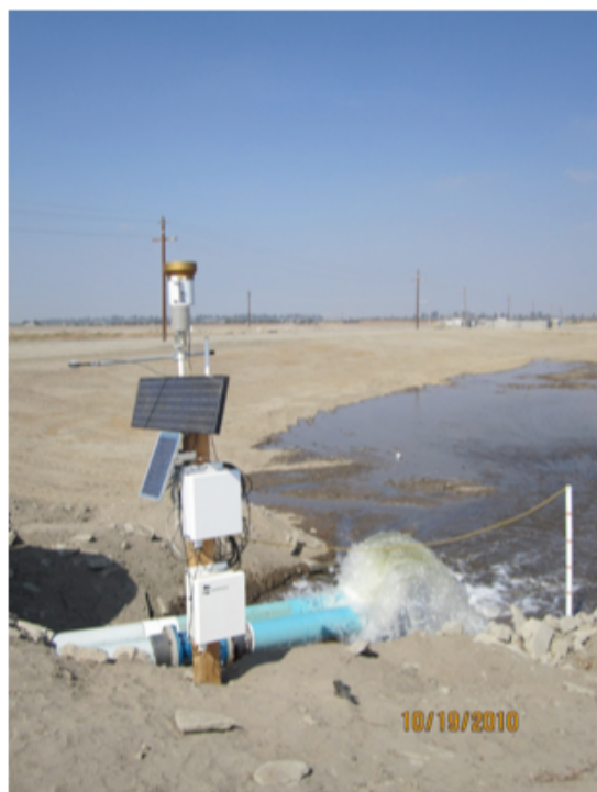
Figure 3. The new CENS-CITRIS managed aquifer recharge network (MARnet) prototype presently installed at the Fresno city wastewater treatment facilities.
